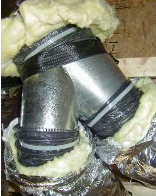
INCORRECT: No Mastic
