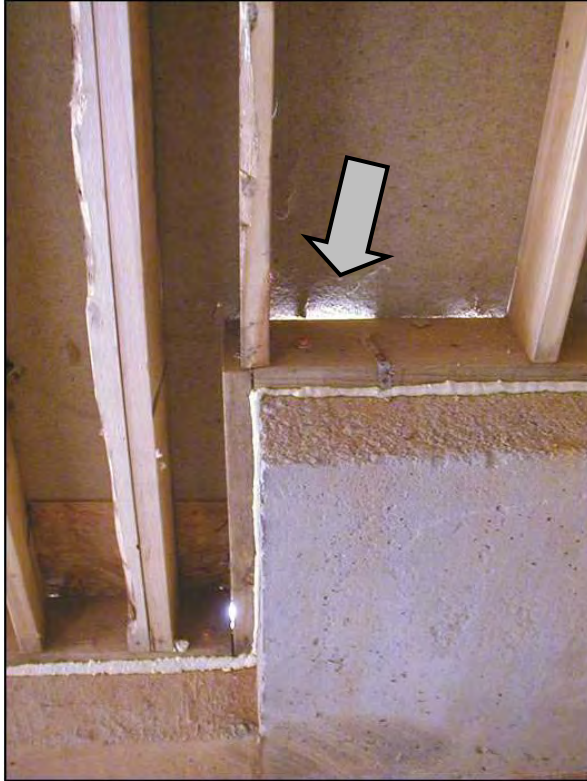
INCORRECT: Gaps in Sheathing
