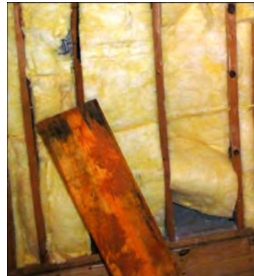
INCORRECT: Unfilled Cavity
