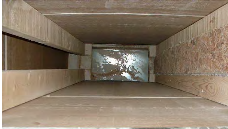
INCORRECT: Unlined Cavity as Plenum
