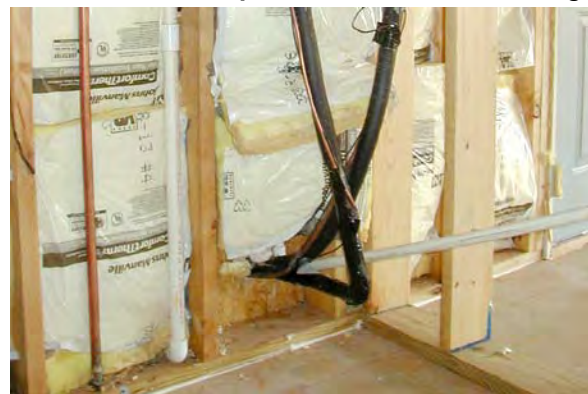
INCORRECT: Compression and Poor Coverage
