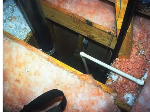
INCORRECT: Unsealed Chase
