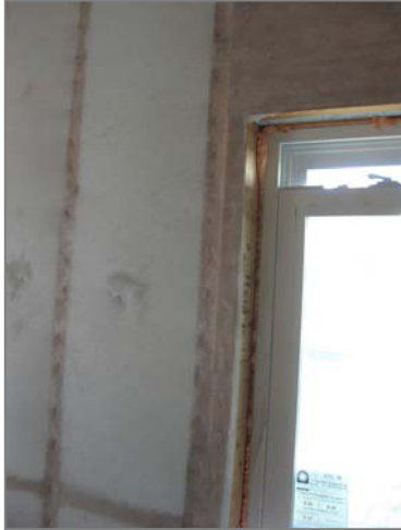
Blown-in cellulose is inspected during the insulation inspection of a multifamily building in Savannah. The NFRC sticker and air sealing around the window were inspected.
