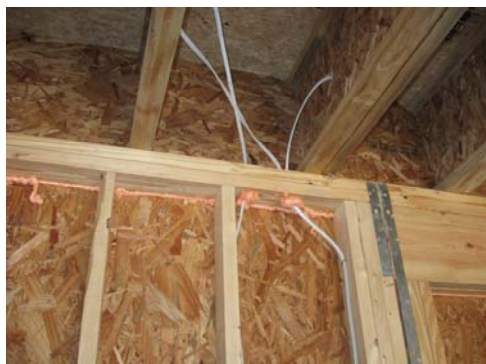
Sealing of framing and wall top plate can be seen on a new home under construction in Chatham County.
