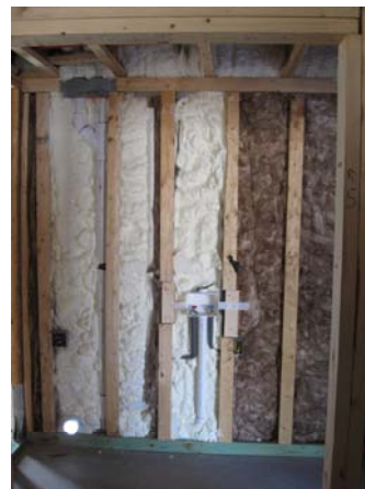
The laundry room wall of this new Chatham County home is sealed with fiberglass batt and spray foam insulation.
