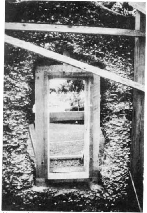
New wood framing at the slave hospital at Retreat Plantation, Saint Simons Island, Georgia.
