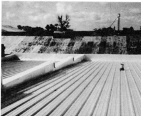
New roofs compatible with the historic character will protect dozens of historic buildings in Plains for many years.
