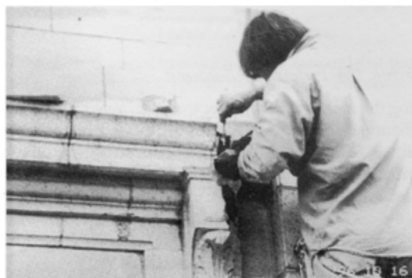
The Flood Recovery Program made it possible for owners to hire skilled craftspeople to rehabilitate their historic properties.
