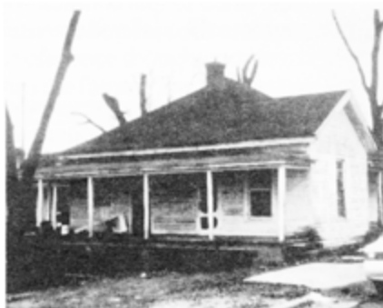
The Ables Residence in Buena Vista was in need of total rehabilitation.
