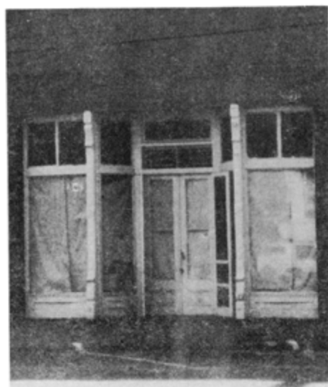
Empty and flood damaged stores illustrate the difficulties Lumpkin faced in the summer of 1994.
