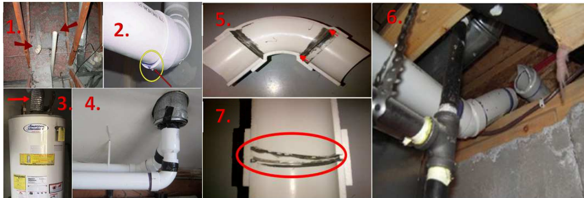
Figure 2: Improper Installation and Installation Related Failures
