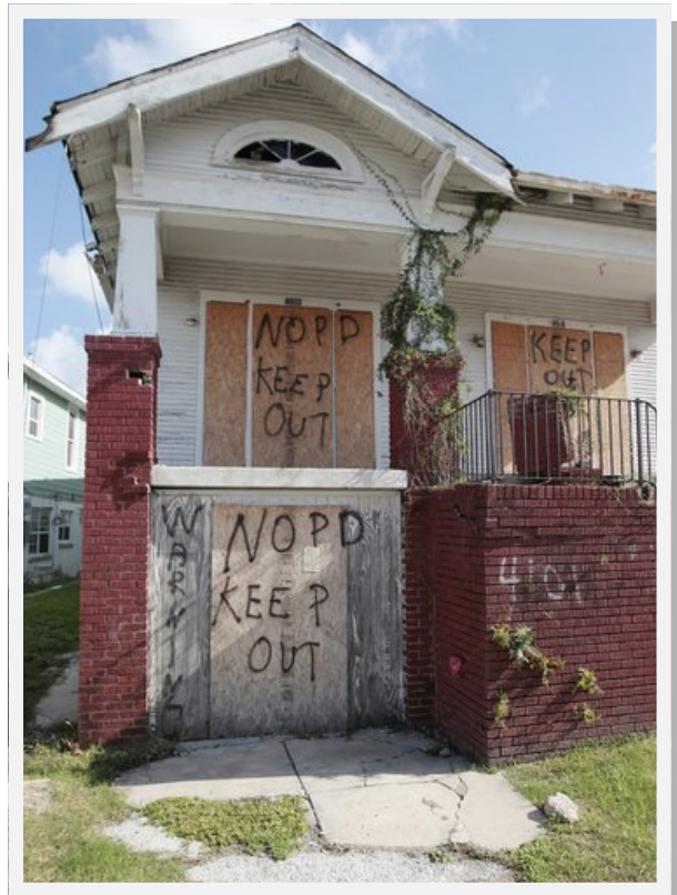
Neglected maintenance can lead to neighborhood blight
