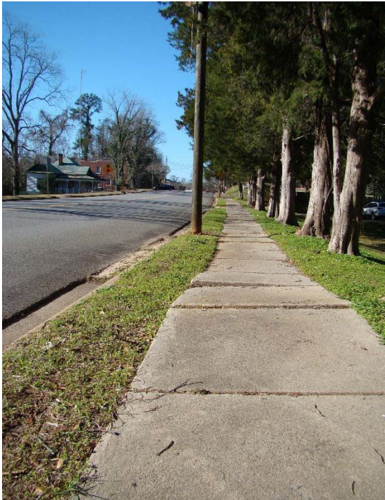
Figure 10 – A damaged sidewalk in Irwinton to be repaired with a forthcoming grant.
