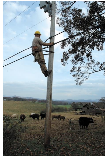
Telecommunications tech working on infrastructure in rural Northwest GA. Photo courtesy of Ellijay Telephone Co.
