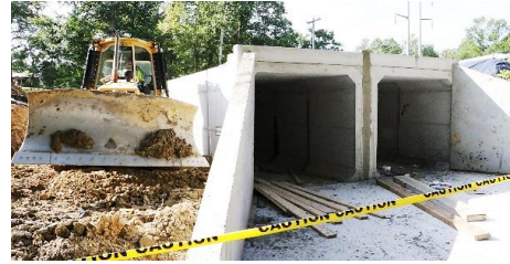
Before and after of a culvert replacement on Beaverdale Rd. where Whitfield County saved approximately $300,00 by utilizing its on public works department rather than a contractor
