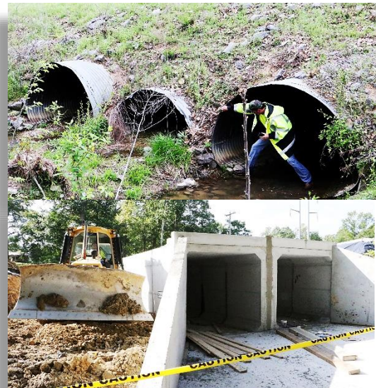
Figure 36: Before and after of a culvert replacement on Beaverdale Rd. where Whitfield County saved approximately $300,00 by utilizing its on public works department rather than a contractor
