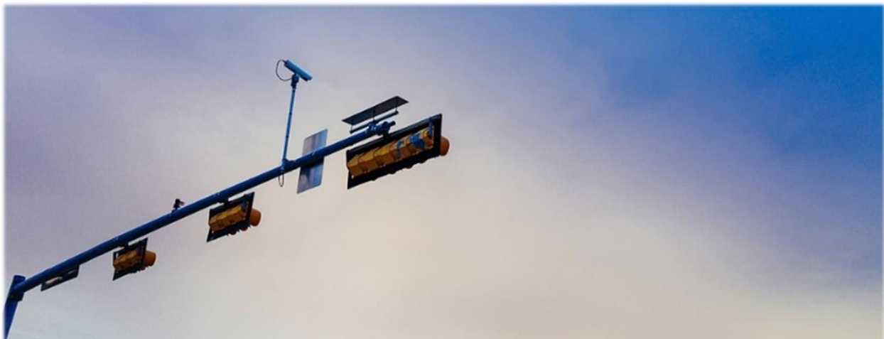
Figure 55: Example of an ITS equipped traffic light
