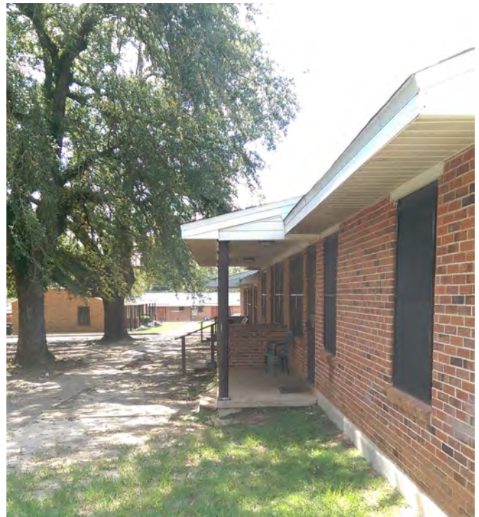
Porches are too shallow to be effectively used by residents.
