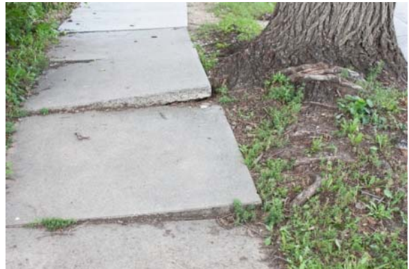
Figure 2: Depicts the sidewalk infrastructure problems.
