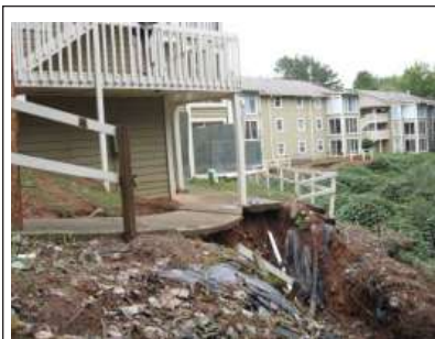
Erosion caused by flooding
