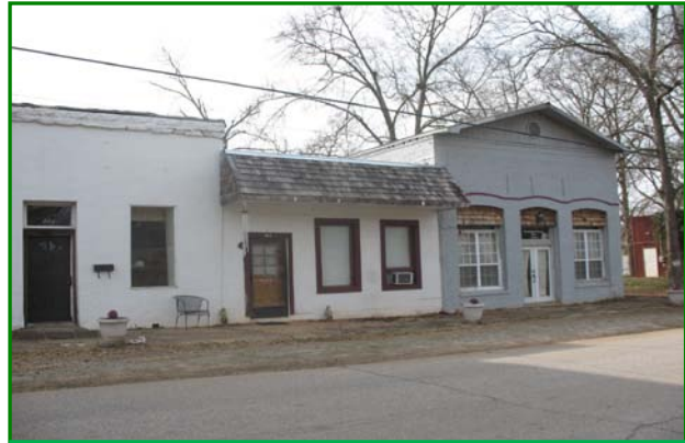
Downtown buildings in need of renovations
