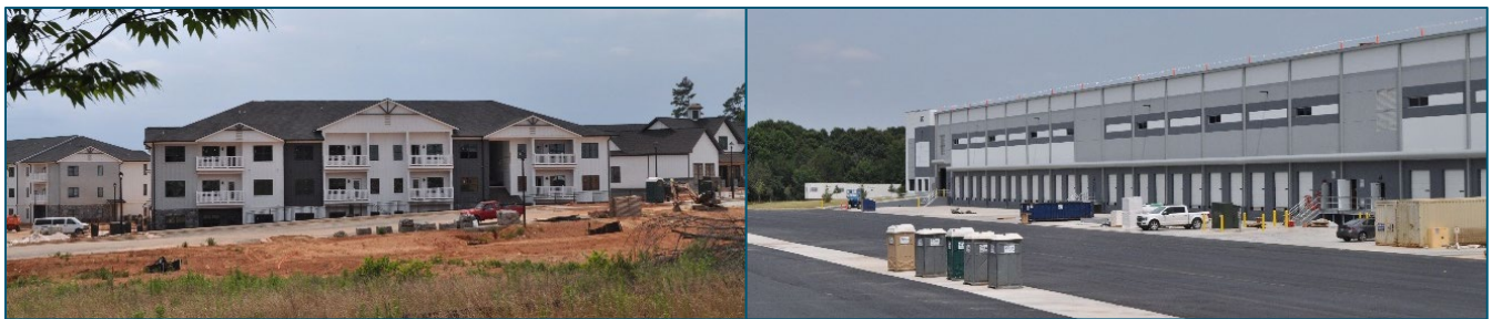
Figure 11. Construction is currently underway on several industrial and residential developments, including warehouses, single-family residential neighborhoods (not pictured), and Pendergrass’s first multi-family housing complex.
