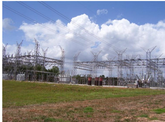
Power Substation on SR 334
