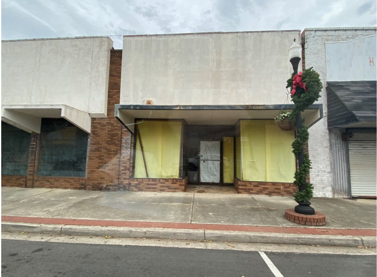
Photo 14: Abandoned storefronts in downtown Fort Valley (MGRC Staff Photo)
