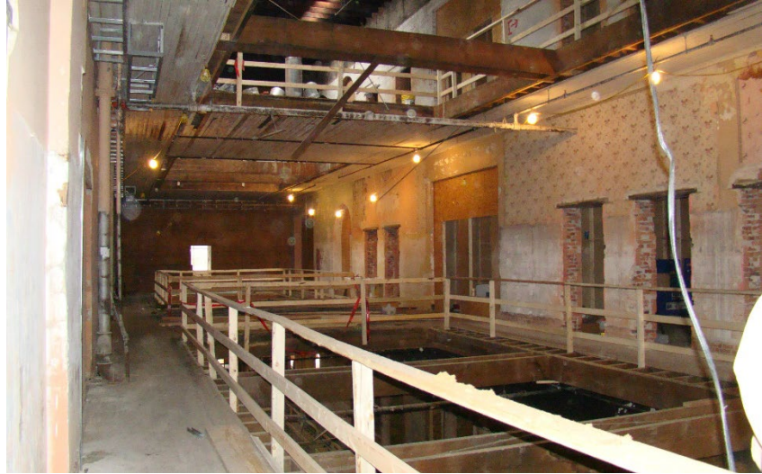
Photo 10: Dannenberg Lofts in downtown Macon, during redevelopment. The building became a catalytic mixed-use redevelopment. (MGR Staff Photo)
