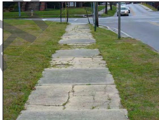
Sidewalks cracks and encroaching vegetation along Tom Watson Way
