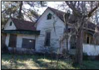
Dilapidated House in Ludowici
