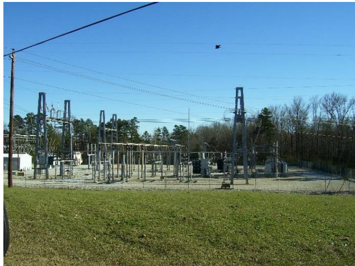
Electric Utility Substation
