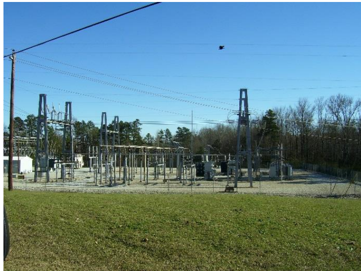
Electric Utility Substation
