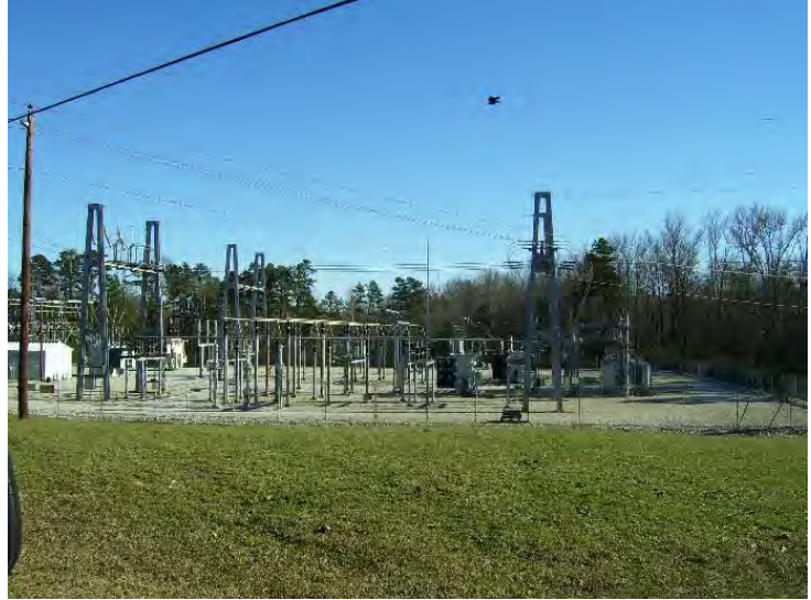
Electric Utility Substation
