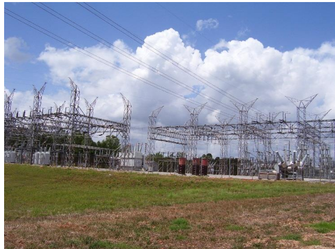
Power Substation on SR 334
