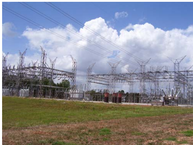
Power Substation on SR 334
