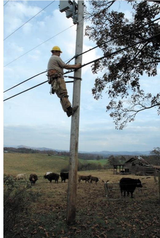
Figure 46: Telecommunications tech working on infrastructure in rural GA. Photo courtesy of Ellijay Telephone Co.
