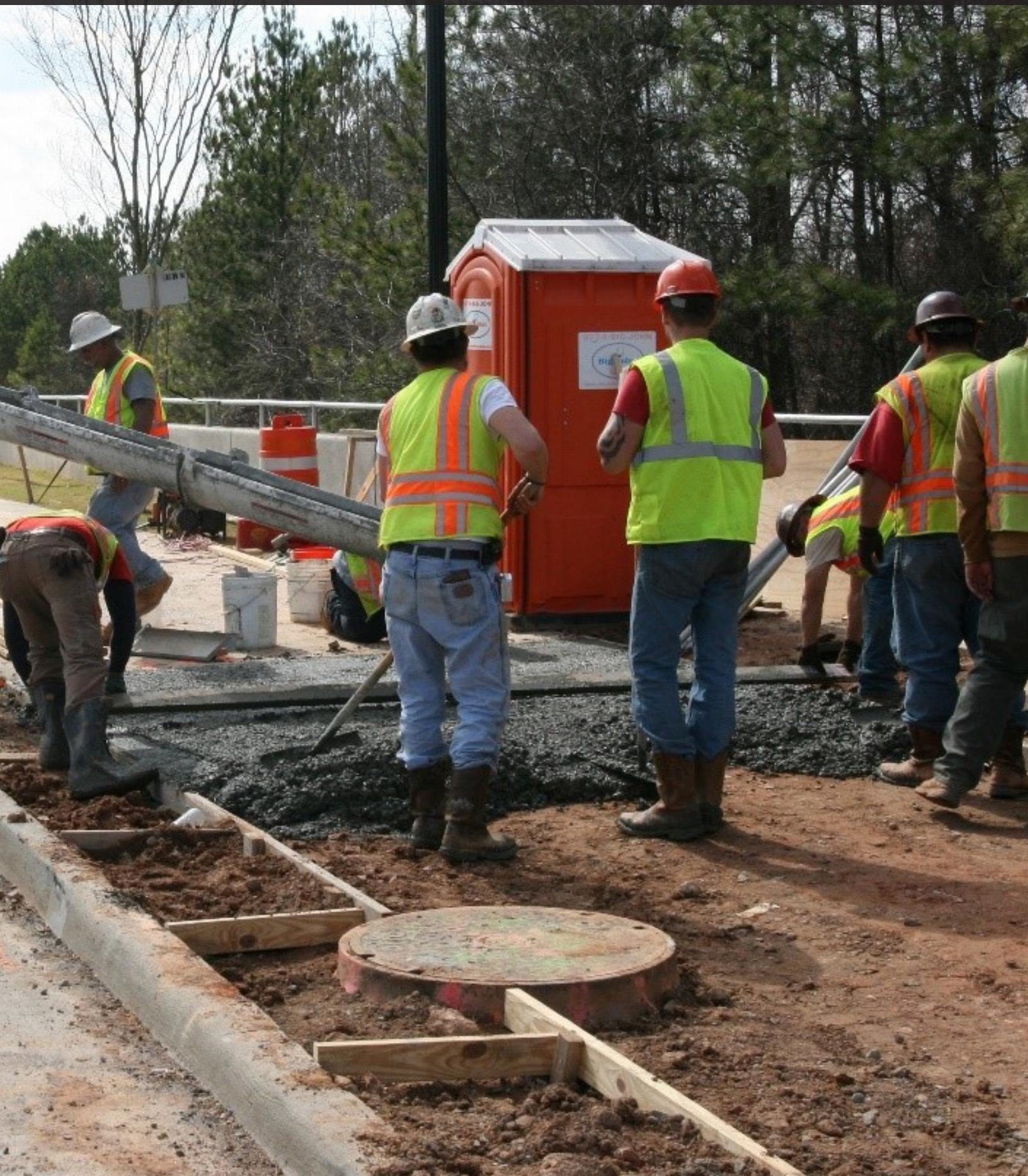
A Gwinnett County DOT construction crew installs new sidewalks at the intersection of Sugarloaf Parkway and Satellite Boulevard
