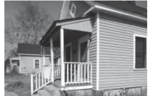
The shotgun house, such as those in Americus (above), is a working class housing type that dates from the 1890s to the 1930s. This house type is an endangered resource that has been "rediscovered" in urban areas.
