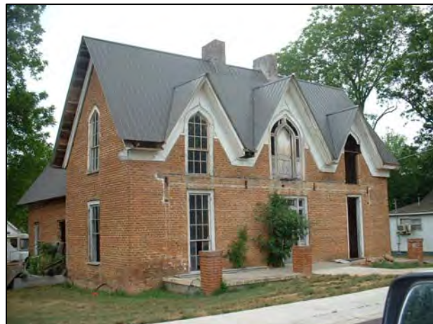
Existing and former residential uses are also found in the downtown area, including this historic structure in need of repair
