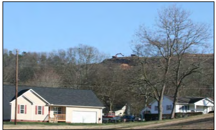
Breaking ground in Fairmount: Construction of a 600-lot residential development is evident beyond the existing homes shown in the foreground
