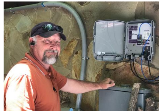
Figure 54: ETC technician installing residential phone and internet infrastructure. Photo courtesy of ETC.
