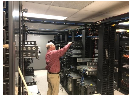
Figure 52: ETC technician working on a large server. Photo courtesy of ETC.
