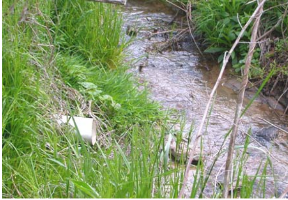
This straight pipe discharged household sewage directly into a stream. A new septic system was installed as part of a voluntary grant program.
