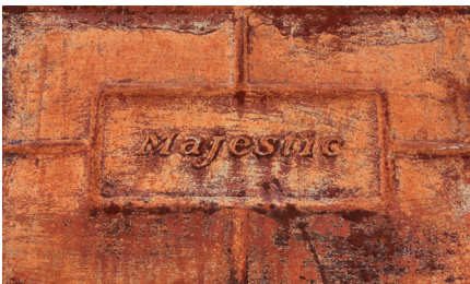
Image 14: Rusted vent on a high school gymnasium
