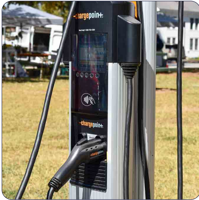
Image 13: Free to use EV charging station
