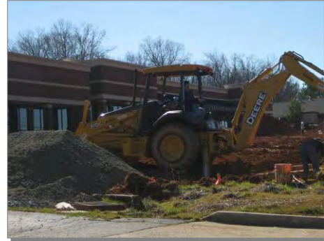
New strip commercial shopping centers under construction on Atlanta Highway in Auburn
