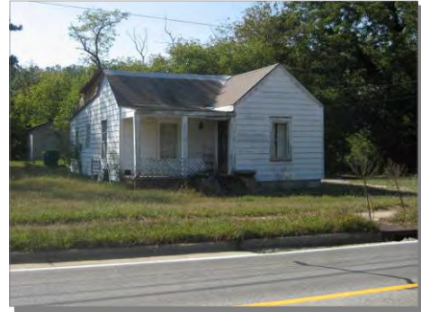
Typical single-family home in disrepair in Carl's Transition Corridor
