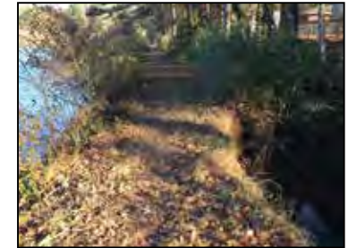
Pending failure of Twin Brothers Lake shoreline
