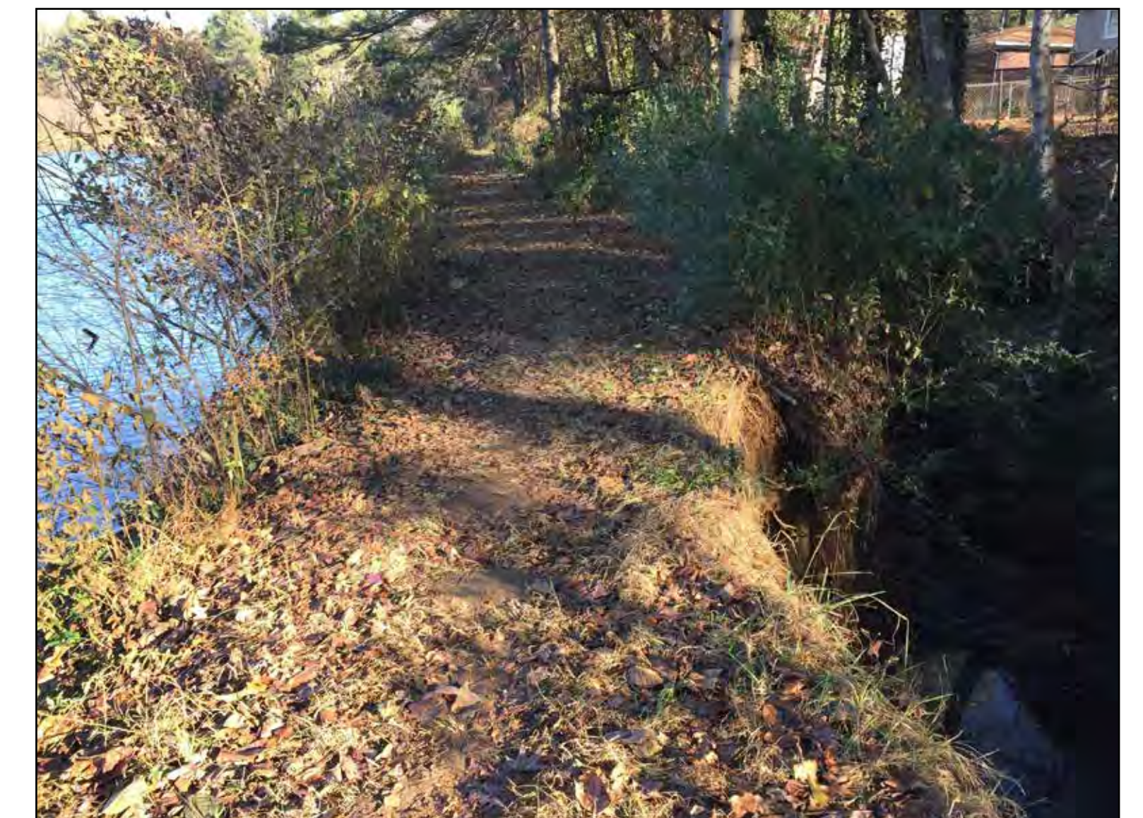
Pending failure of Twin Brothers Lake shoreline
