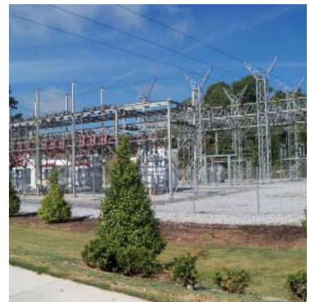
This power substation is classified as TCU-utilities.
