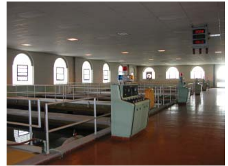
Interior of the Hemphill Water Treatment Plant.
