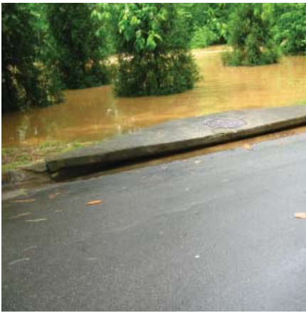
Flooding along the right-of-way.
