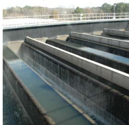
Sand Filters at the RM Clayton Plant.
