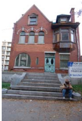
A single family home in poor condition, NPU M.
