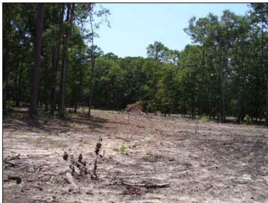
Forested land in St. Marys is cleared to make way for residential opportunities.
