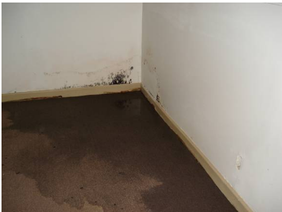
Water and mold in a vacant unit
