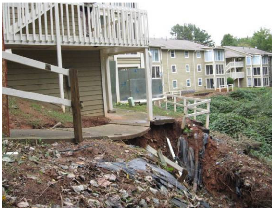
Erosion caused by flooding
