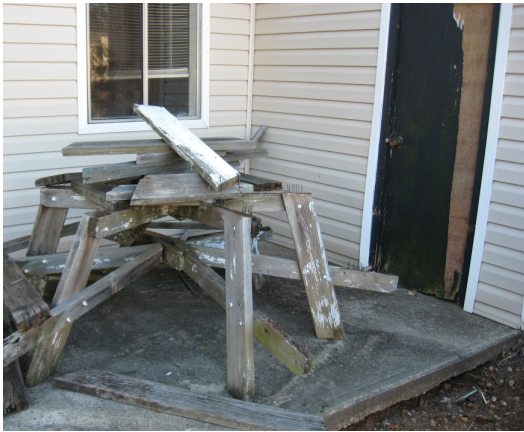
Debris, shearing under pad, rotten door
