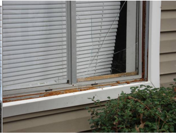
Broken window and rotting sill
