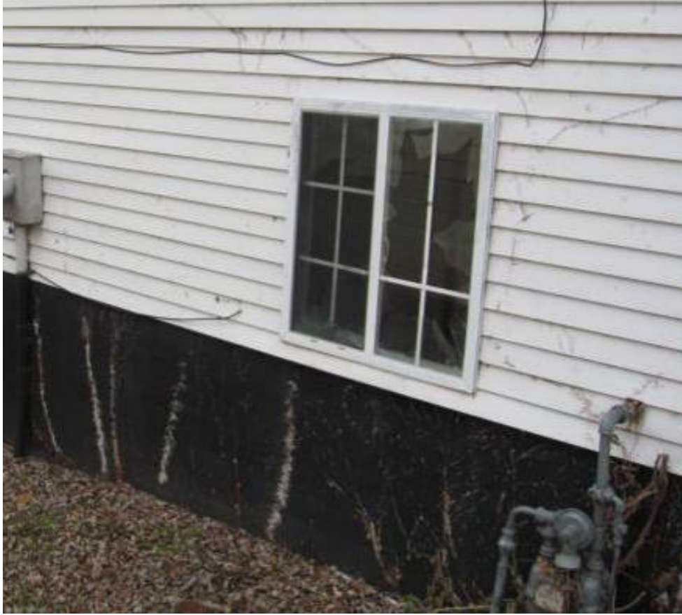
Broken basement window, vines removed
