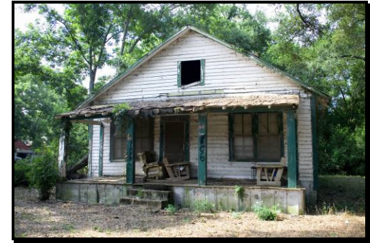
Dilapidated, Abandoned Home
