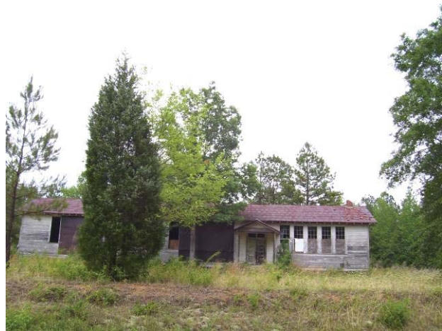
Historic Structure that Suffers from Neglect
