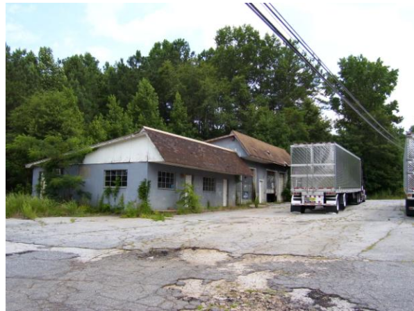
Opportunity to revitalize an obsolete commercial property along Homer Road (U.S. Highway 441 Bus.) for neighborhood commercial
