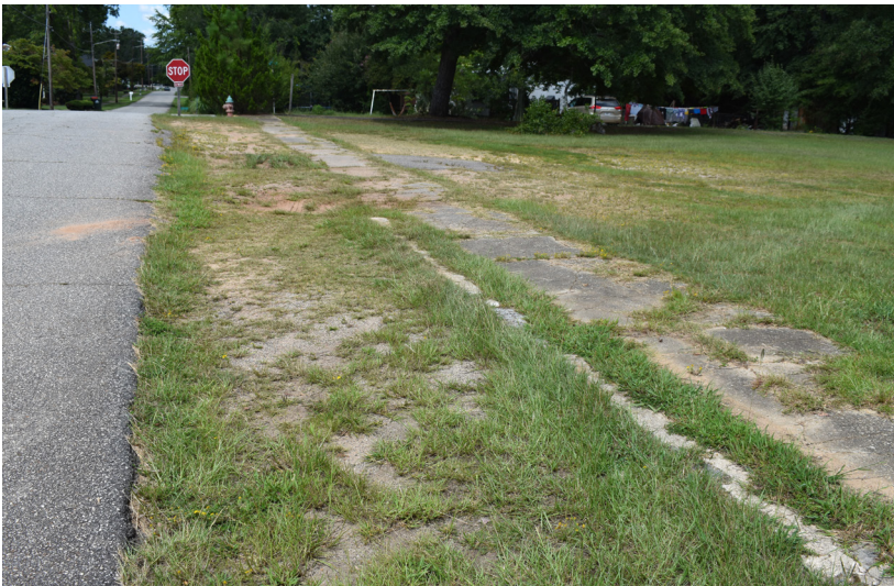
Figure 4. Sidewalks are found throughout the historic downtown (top) and are required in new developments. In much of the rest of the city, sidewalks are either missing or are in disrepair (bottom). In addition, many sidewalks, like those pictured, are difficult to use on hot days due to the lack of shade.
