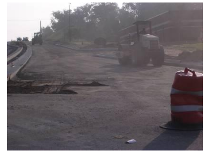
The construction of new roads should be balanced with the maintenance and improvement of existing roads.
