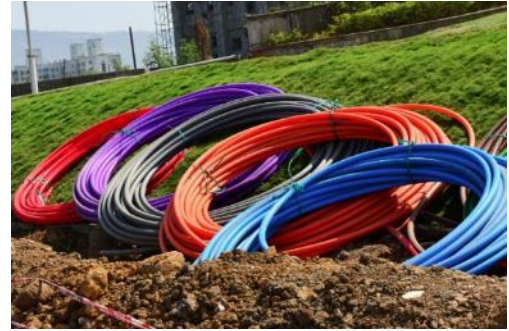
Modern broadband technology relies primarily on terrestrial-based infrastructure such as fiberoptic cable, shown above.
