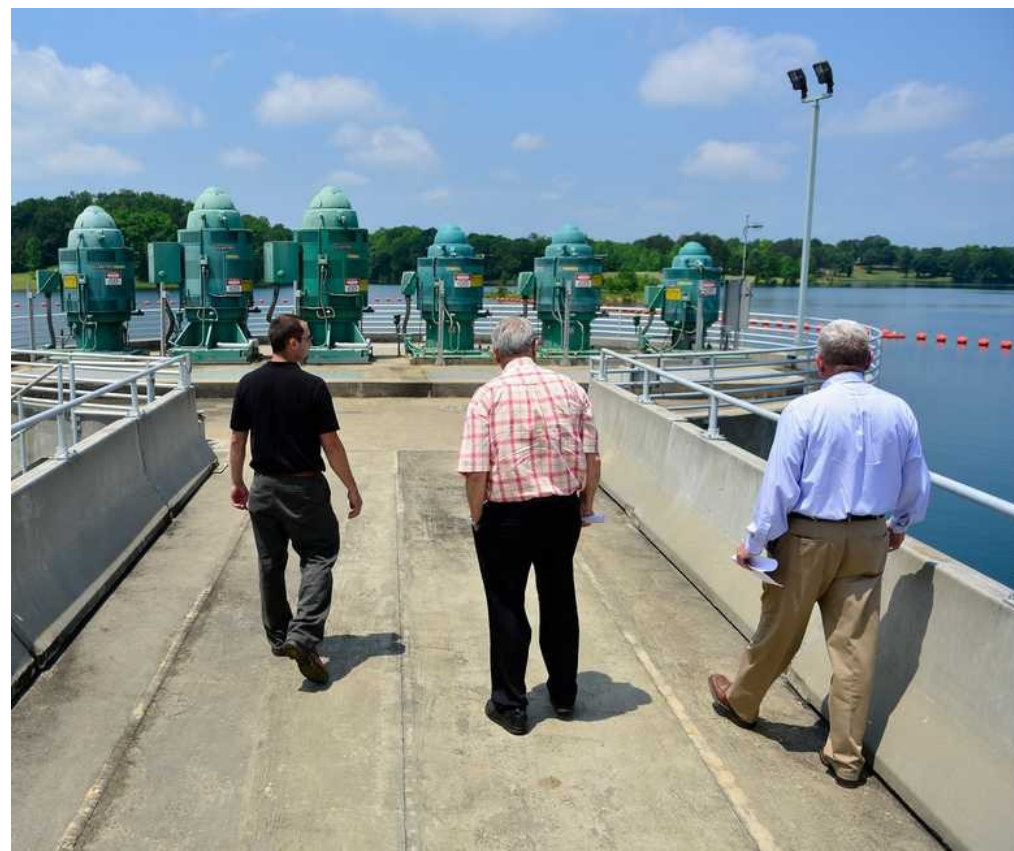
Bear Creek Regional Reservoir & Treatment Plant
