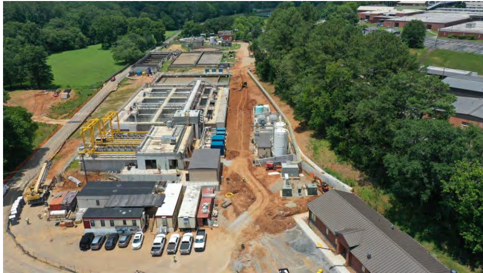
Canton Water Pollution Control Plant
