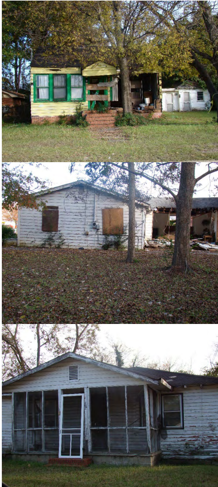
Photo 11: Several homes identified in a 2018 application by the City of Fort Valley for housing rehabilitation assistance
