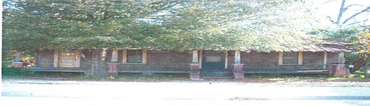
Substandard home on MLK Jr. Blvd.
