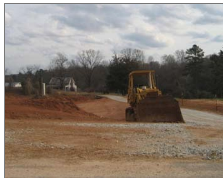
Bulldozer shown above working to prepare land for new development near I-85
