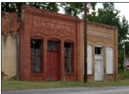
Historic buildings in need of repair in Vidette
