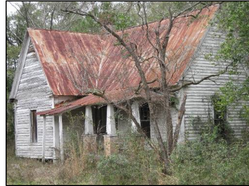
Substandard historic house standing in Girard
