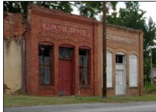
Historic buildings in need of repair in Vidette
